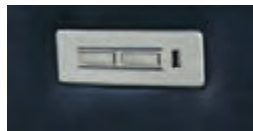
9) Detail Control Panel
