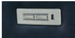
9) Detail Control Panel
